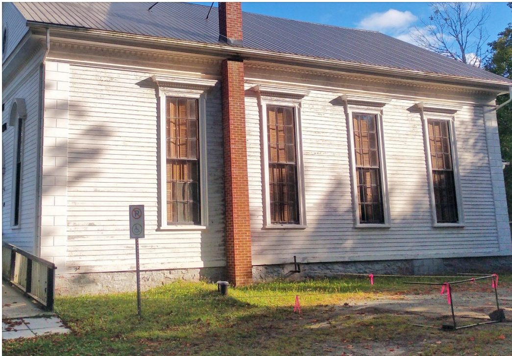
Chimney at side of former church, showing wellhead and parking area (including accessible parking) roped off due to risk of collapse
