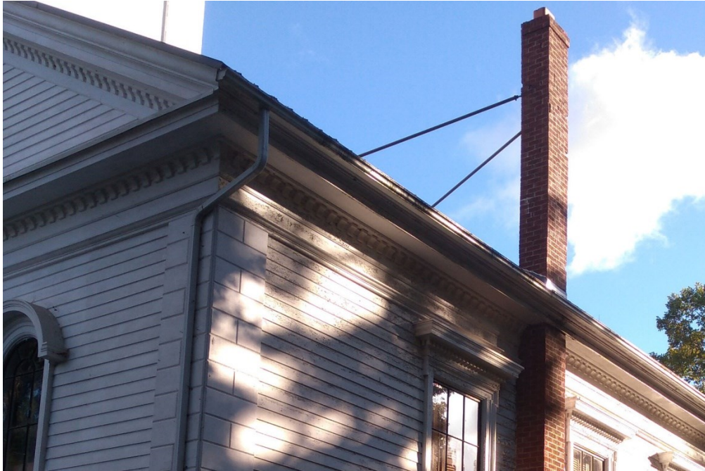
Outward bowing of chimney suggests potential for failure
