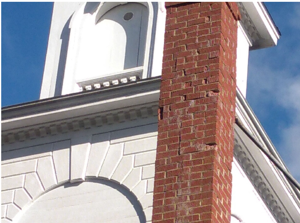
Horizontal and vertical cracks, mortar loss, and corner failure on upper chimney above roof
