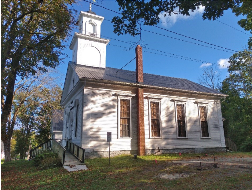
High Tides Arts and Culture Centre (former St Davids's United Church), built 1858, showing location of chimney along north side elevation
