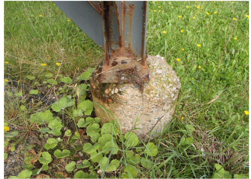
Photo A8 - Base plate corrosion and deteriorating concrete pier
