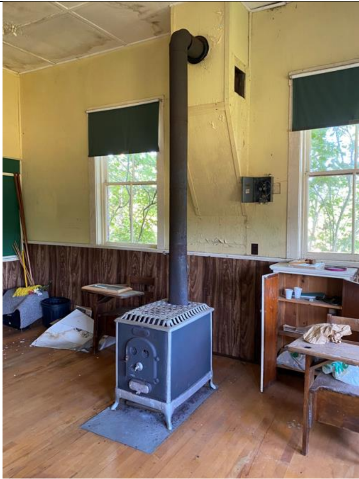
View of heating system (uncertified wood stove) and electrical panel (no power, requires upgrade)
