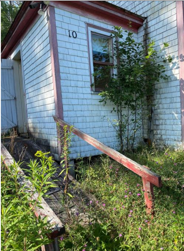
View of entrance ramp; evidence of wood rot and overgrown vegetation
