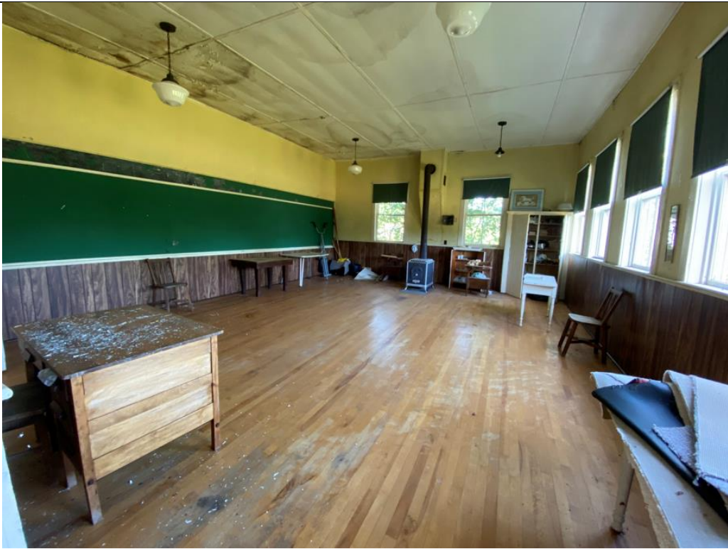
Interior view; evidence of water damaged building materials
