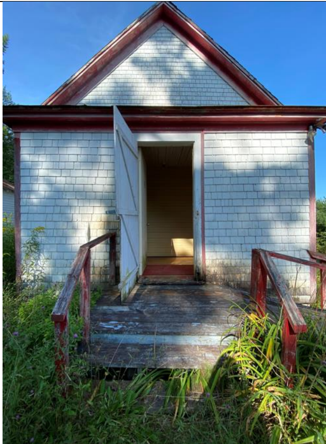
View of entrance steps; evidence of wood rot and overgrown vegetation
